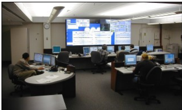
Figure 3: New space showing ergonomic workstations and main DLP display wall. Remaining equipment racks are in upper left corner.
